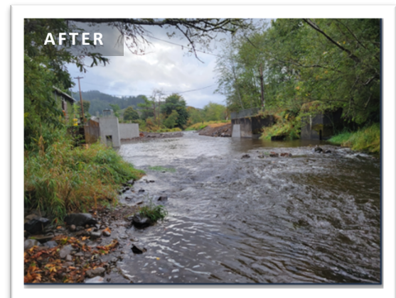
AFTER: Wild fish will have unimpeded access during times when the inflatable replacement weir is lowered. During operation, there will be a functional fish ladder and passage facilities to allow for unimpeded upstream lamprey and juvenile salmonid volitional movements. Full year, downstream juvenile fish migration will be improved for all species.
