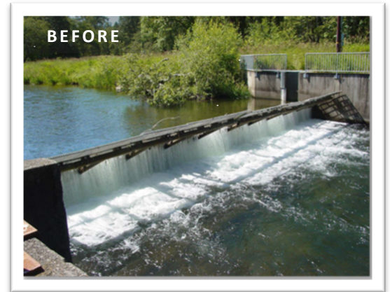
BEFORE: The channel spanning weir at the Cedar Creek hatchery on Three Rivers was impeding fish passage to over fourteen miles of habitat.
