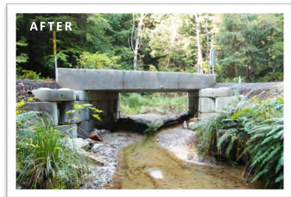
AFTER: The new bridge crossing provides safe access for residents Boy Scout campers, and restores full access to 0.75 miles of habitat for fish and other aquatic organisms.
