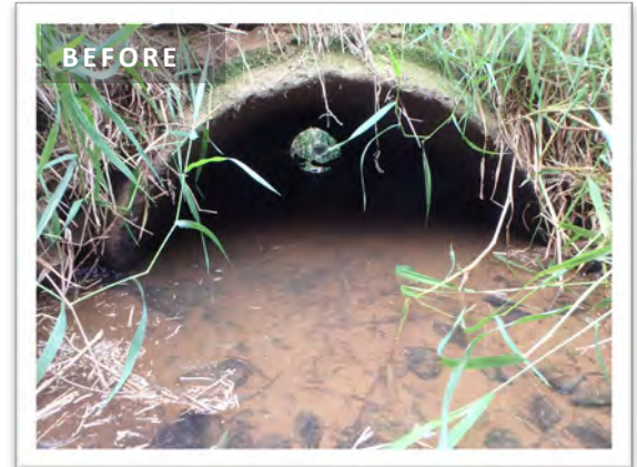
BEFORE: One of three deteriorated culverts.
