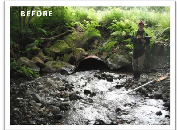
BEFORE: The undersized culvert at Mapes Creek required constant inspection and maintenance to prevent plugging and overtopping.
