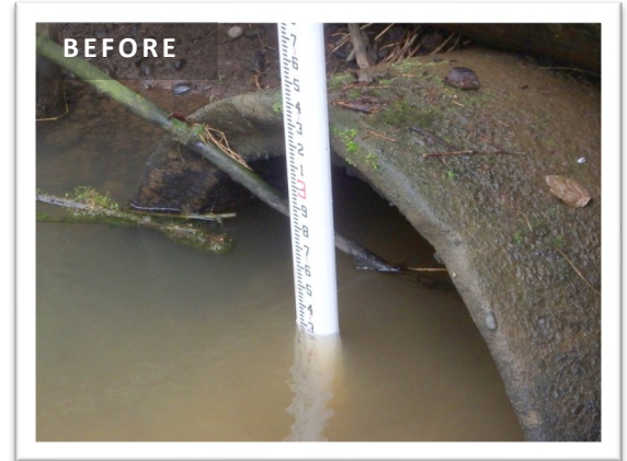
BEFORE: The culvert at Chance Creek was very undersized, was prone to clogging, and impeded fish passage to upstream spawning and rearing habitats.
