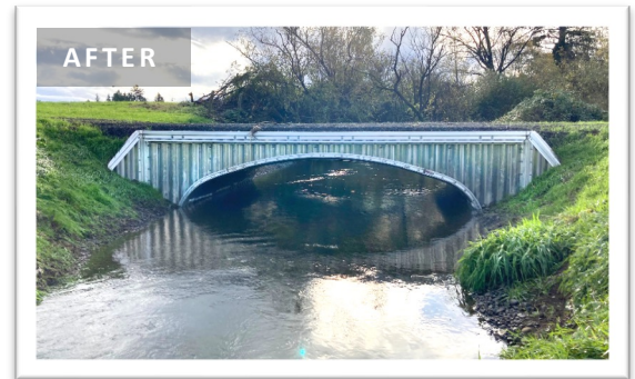
AFTER: The new culvert enables conveyance of high flows, and restores full volitional fish passage at this location in Chance Creek.
