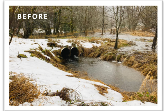
BEFORE: The culverts at Alder Creek were prone to clogging and impeding passage to several species of native migratory fish.
