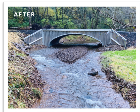
AFTER: The new bridge provides full volitional passage to five species of fish, and restores natural stream processes including transport of sediment, wood, and high storm flows.
